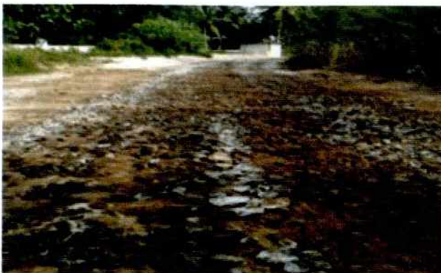
View of mine haul road after laying coir pith & coarse aggregate and 33% calcium chloride
