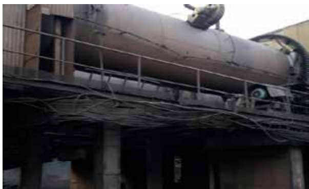
View of 50 TPD capacity commercial DRI Rotary kiln used for metallisation of ilmenite
