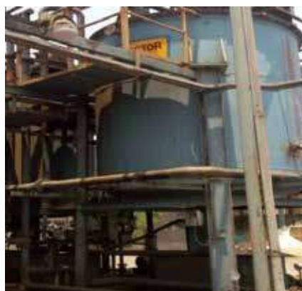
Photograph of rusting reactor
