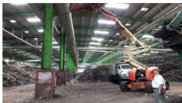
Gas biofilters under construction at 500 tpd municipal solid waste treatment facility. Installation of exhaust ducting.
