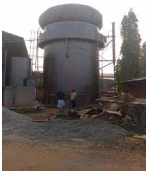
Effluent treatment plant with BFBR anaerobic reactor at Keerthi Rice Mill, Kalady installed by NIIST licensee: Galaxy Environ Pvt. Ltd.
