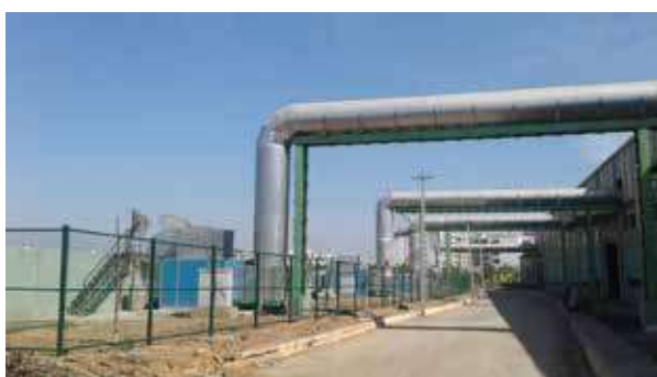
Odour control system at 500 tpd MSW mechanical biological treatment plant at KCDC, Bengaluru.
