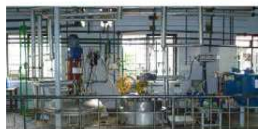
Unit operations in the Biofuel Pilot Plant
