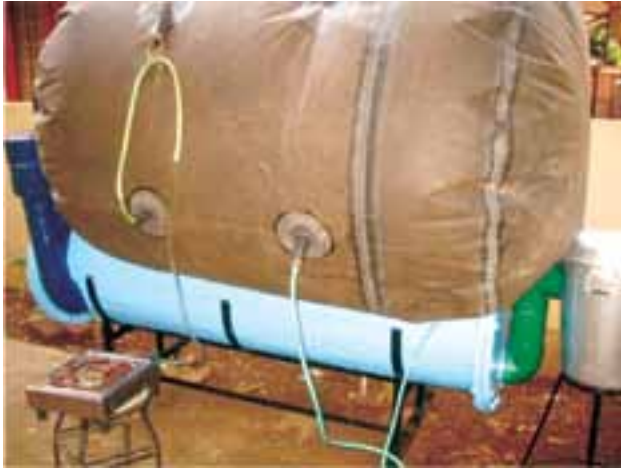
Household Wastes Digester cum Biogas plant
