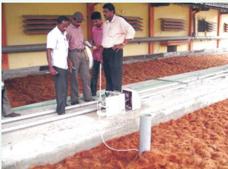
Testing efficiency at odour control gas biofilter treating 34,000 m 3 /h air from meat meal factory.
