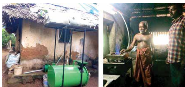
Small capacity NIIST digester installed at a farmer house for recovering biogas from cow dung.
